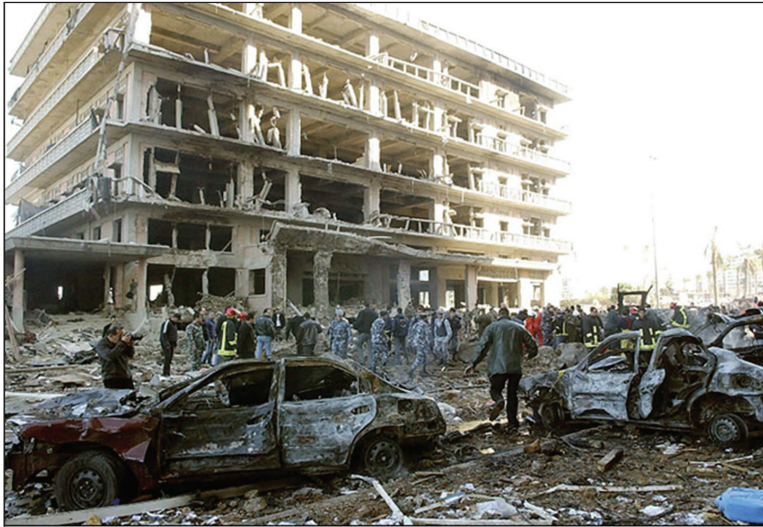
Fig. 3. Damage of Saint-George hotel as the result of the car bomb that killed the Prime Minister Rafik Hariri on 14 February 2005
