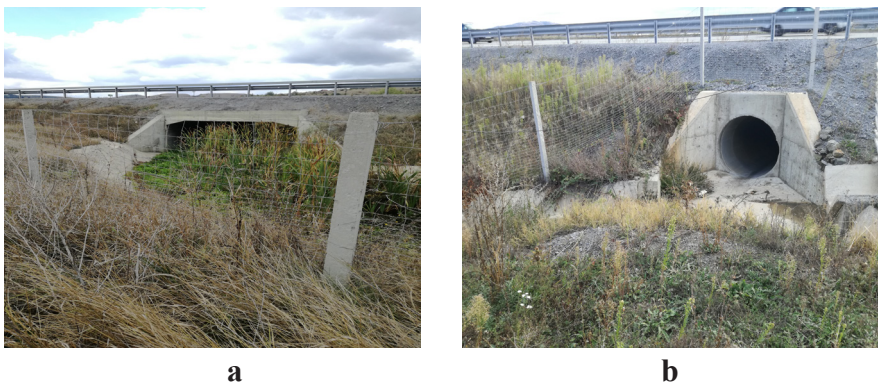
Fig. 3: a) bad implementation of the “rabbit fences” at the bridges; b) good implementation of culvert with guiding fences;
